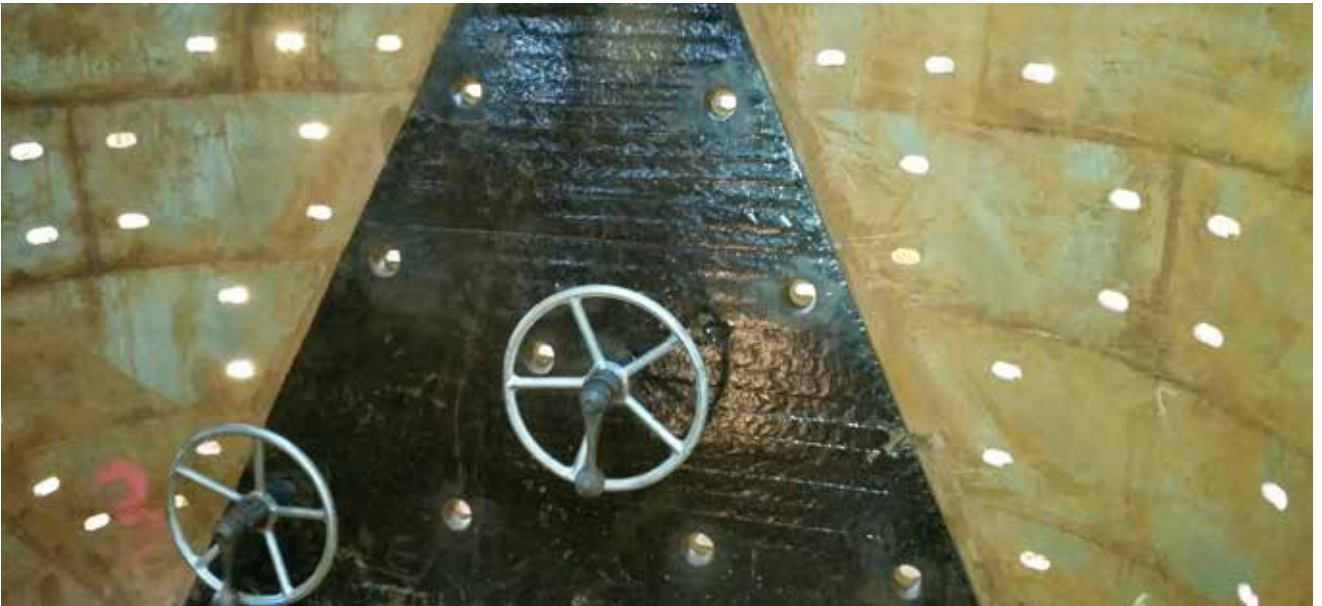
SafeFit clamps holding a liner in position awaiting the installation of Taper-T attachments.
